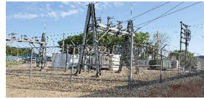
Figure 15 Electric Utility's Industrial Substation
